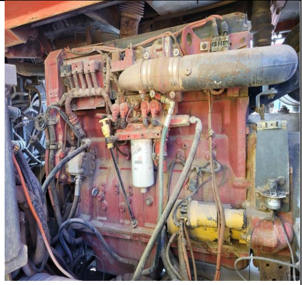
Diesel engine looks in good condition and has no leaks
