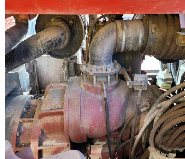
Compressor status normal and without leaks
