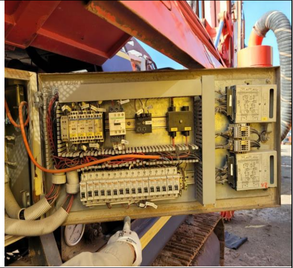
Main electrical box in good condition
